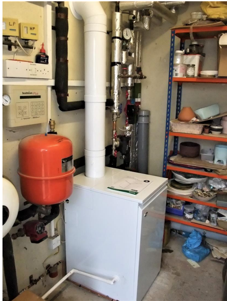
New Boiler at Llanishen Village Hall
